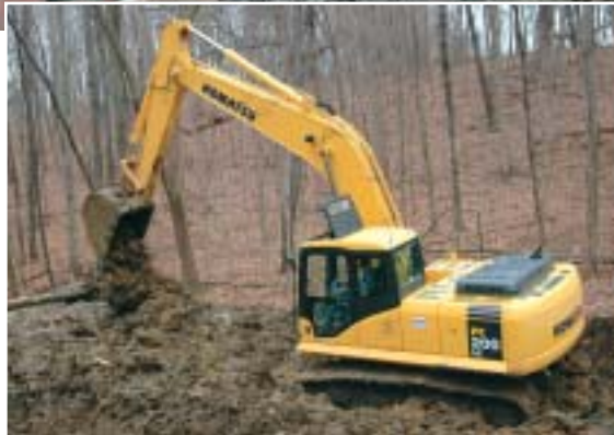
Valley Construction also put its Komatsu PC200LC-7 excavator to work at the Rapids City sewer line project.
