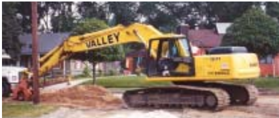
A Valley Construction operator uses a Komatsu PC200LC-6 excavator on a residential utilities job.
