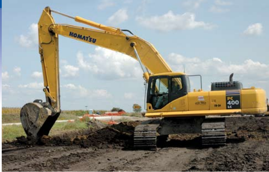
Eco-Tech uses several Komatsu excavators, such as this 96,712-pound PC400LC-7, for utility installation, concrete removals and mass excavation. The company also has four PC200LC-7 models. "We've found that they will outperform the competition in the same size class," said President Doug Jones. "The PC400 has been especially good for concrete removal and digging ponds. We've found them to be excellent machines."
